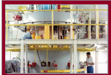
K500 SUPERCONDUCTING CYCLOTRON (1987) The Cyclotron Institute at Texas A&M University operates one of only five K500 superconducting cyclotrons in the world.
